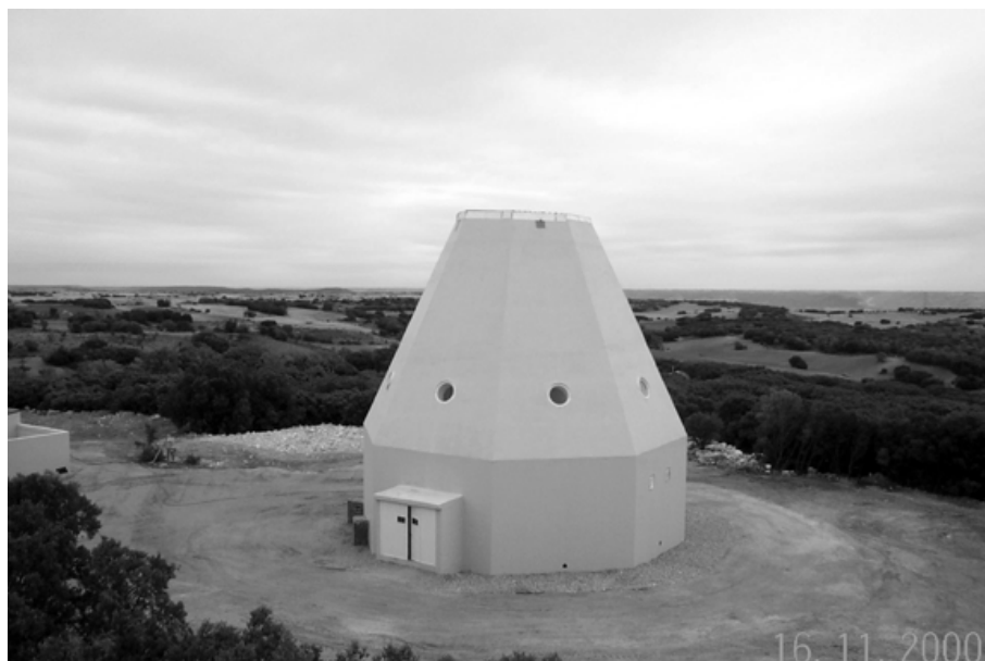
Figure 2. Status of the construction of the new 40 meter radiotelescope of OAN at Yebes (Guadalajara, Spain). The finished concrete pedestal is shown.
