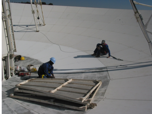
Figure 2. All upgrade work to the telescope surface is done on site by our own staff. Here Amos Kekae and Jacques Grobler are working on the installation of new panels.
