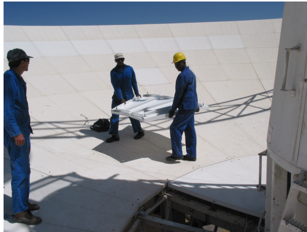
Figure 1. The last panel of the 26 metre radio telescope surface upgrade being installed by Simon Morake and Andrew Masiteng.
