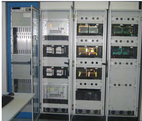
Figure 1. Left-most rack contains the two correlator crates. Rack second from left contains two station units with two rack-mounted Mark 5A playback units. Rack second from right contains from top to bottom three Mark 5B units and the eVLBI-dedicated linux computer. Right-most rack contains two Mark 5B units.
