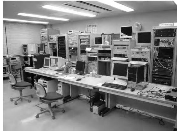
Figure 1. A view of the observation room of the Kashima 34m antenna. The K5 system in this room is used both for observation and correlation processing.
