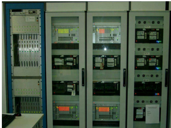
Figure 1. The left-most rack contains the two correlator crates. The racks second and third from left contain two station units with two rack-mounted Mark 5A playback units. The right-most rack contains three Mark 5B units and a Mark 5A unit dedicated for e-VLBI.
