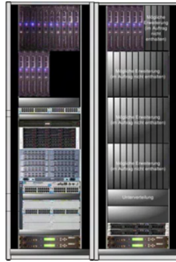
Figure 2. Scheme of the Linux cluster. The left rack contains top to bottom: part of the nodes, the service node (with keyboard and monitor), the 20 TB disk RAID, the switches and the panel control. The right rack contains top to bottom: part of the nodes, empty slots for future nodes and the panel control.
