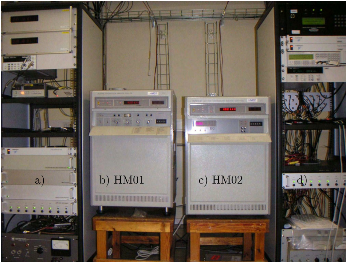
Figure 2. Time lab at Onsala: a) Rack with, for example, GPS TAC, several 5 MHz distributions, pulse distribution unit, b) HM01: Kvarz CHI-75 installed in March 1997, c) HM02 Kvarz CHI-75A installed in April 2007, d) Rack with, for example, GPS time receivers, AOG (Auxilliary Output Generator) for UTC generation, and space for the Cesium clock (to be installed during 2008).
