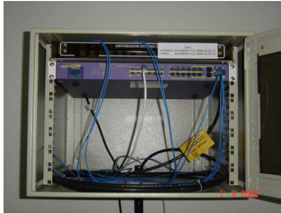
Figure 3. Switch rack for connection to the high speed fiber network.
