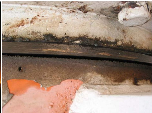
Figure 2. The 26-m telescope breaks down. The gap between the bearing housing and static ring confirms suspicion of a south polar bearing collapse.
