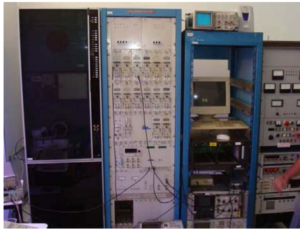
Figure 2. Fortaleza station control rack.
