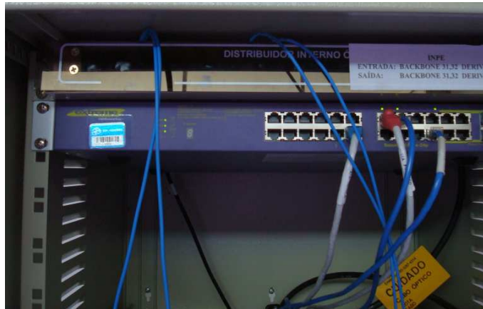
Figure 4. High speed network switch.
