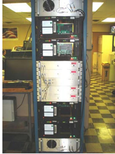
Figure 1. Rack containing a complete VLBI2010 8 gigabit per second data acquisition system. The center chassis contains the optical fiber receivers, splitters, and amplifiers. The four adjacent (silver) chassis with red LED panels are the UpDown Converters. The four black chassis are the Mark 5B+ recorders. The top and bottom chassis are the Digital Back Ends. Each DBE chassis contains two DBE units.
