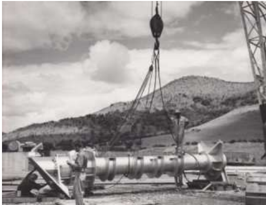
Figure 3. The polar shaft, ready for installation as a 16-ton pre-assembled unit back in 1961.
