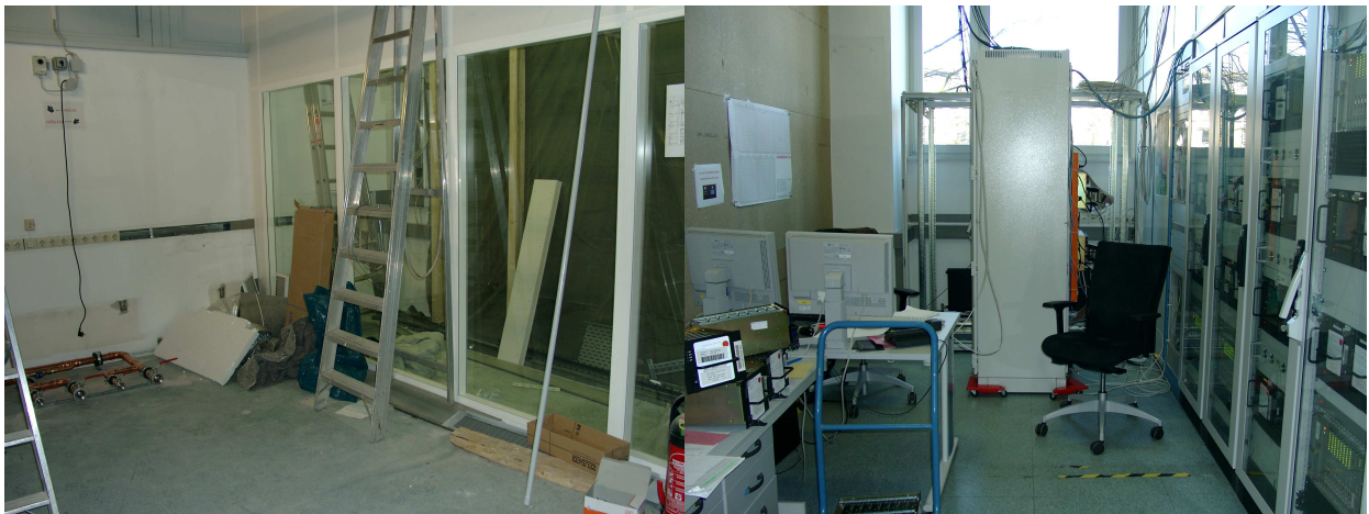
Figure 1. Left picture: sound and thermal insulation room for the software correlator still under construction, right panel: temporary correlator room with one Mark 5A rack (center - side view) standing in-room without cooling.
