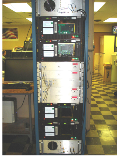
Figure 1. Rack containing a complete VLBI2010 8 gigabit per second data acquisition system. The center chassis contains the optical fiber receivers, splitters, and amplifiers. The four adjacent (silver) chassis with red LED panels are the UpDown Converters. The four black chassis are the Mark 5B+ recorders. The top and bottom chassis are the Digital Back Ends. Each DBE chassis contains two DBE units.
