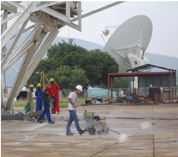
Figure 4. Groundbreaking: cutting the slab for the construction of the 26-m's A-frame support; in the background, the XDM is being put through its paces using the adapted 26-m observing scheduler. (Credit: M. Gaylard)
