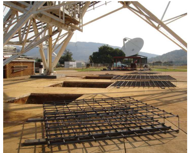
Figure 5. Rebars ready: steel reinforcing bars for the A-frame support's three concrete foundation slabs are ready to go into the ground. (Credit: M. Gaylard)
