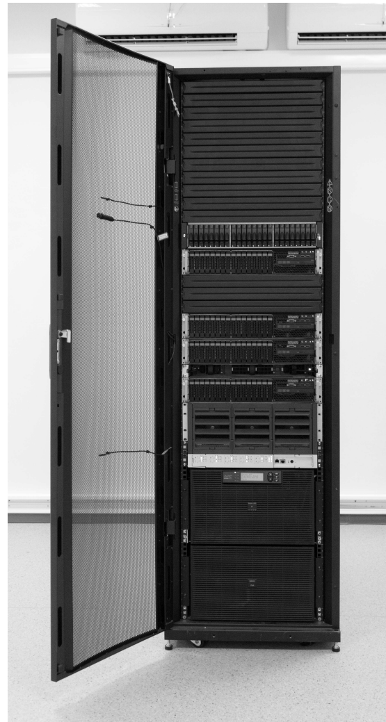
Fig. 2 View of the high-performance computing cluster based on the hybrid blade servers.
