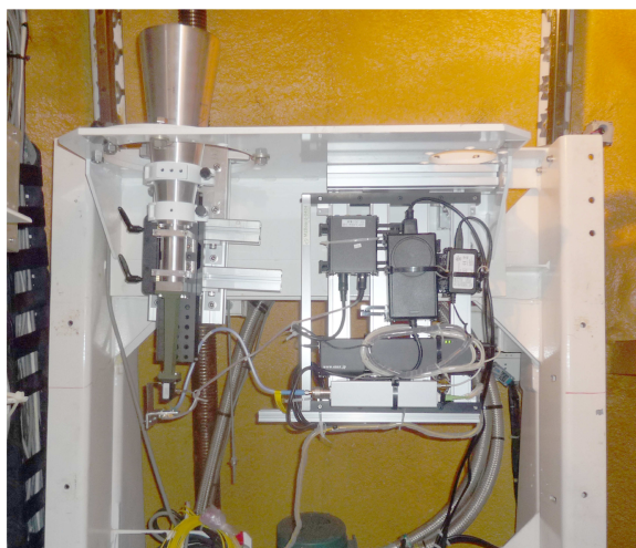
Fig. 2 Broadband (IGUANA) feed installed in the receiver room of the Kashima 34-m telescope.
