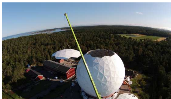
Fig. 1 The replacement of the upper part of the radome enclosing the 20-m radio telescope on 15 September 2014.
