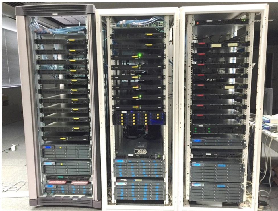
Fig. 2 View of the backup system.
