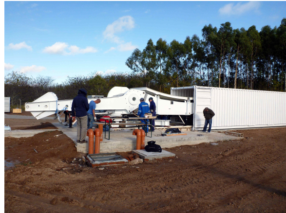
Fig. 3 The re-installation of the former TIGO radio telescope as AGGO radio telescope above a specially constructed platform was performed with the support of the company MT-Mecatronica from Chile (May 6, 2015).
