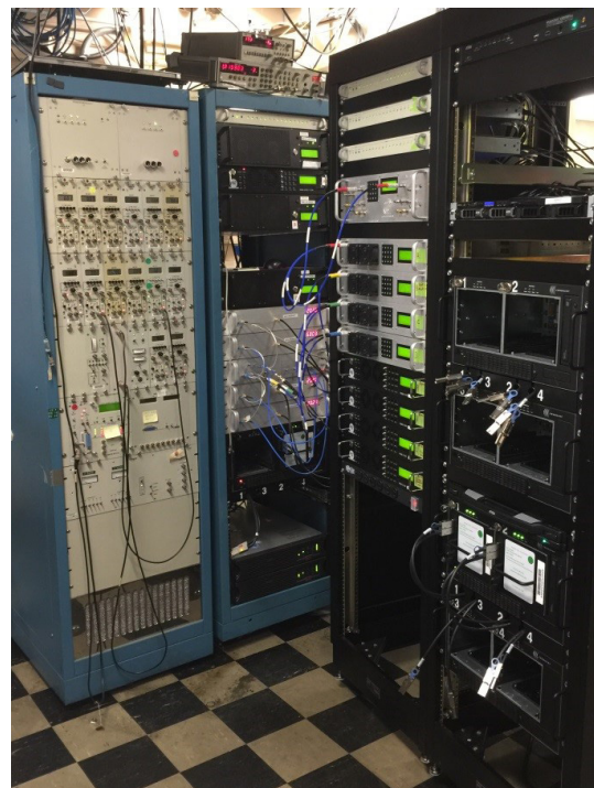
VGOS racks meet legacy Mk4 rack.
