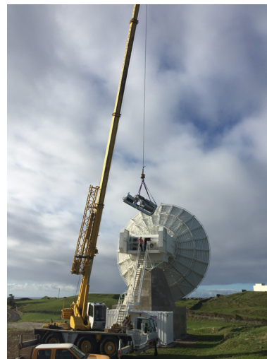
Installation of the tri-band receiver at Santa Maria.
