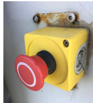
Serious design flaw. The pedestal emergency stop button is at head-height for a kangaroo.
