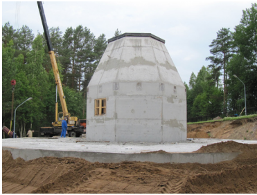
Foundation and antenna tower of the new radio telescope at the Svetloe Observatory.
