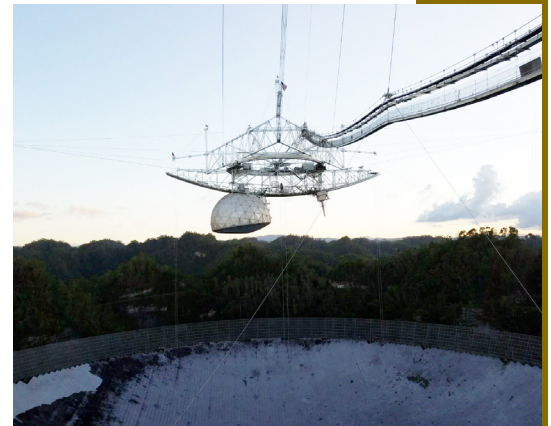
Remaining one fifth of the Arecibo line feed still in place. Photo: Chris Salter/Tapasi Ghosh.
