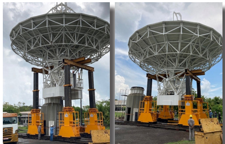
(left) Gantry and Beam System for Lifting; (right) Rolling Gantry and Lowering Antenna.
