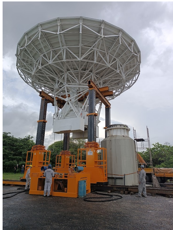
Fig. 2 The 14.2-m antenna set down off the pedestal for bearing replacement activity.
