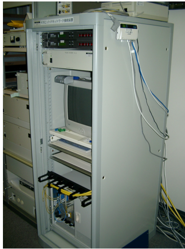
Figure 3. The terminal of Giga-bit IP network
