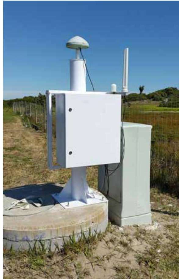
Fig. 6 NMMU GeoStation installation, Port Elizabeth, South Africa.
