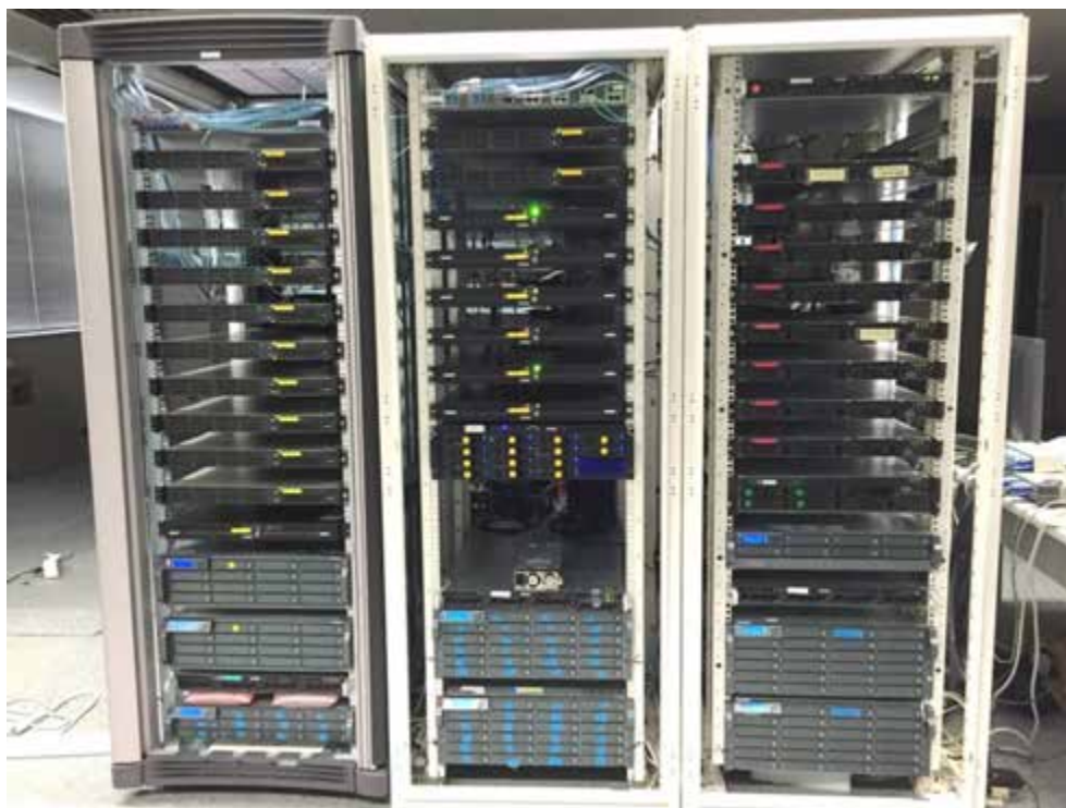
Fig. 2 View of the backup system.
