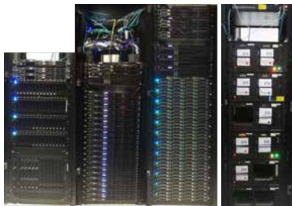
Fig. 2 DiFX cluster system and Mark 5A/B units.
