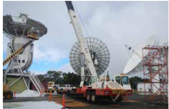
Fig. 4 9-m telescope demolition effort, with the 20-m and the 12-m operating in the background.
