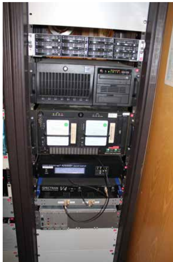
Fig. 3 The new data acquisition rack with (from top) backup system, Field System PC, Mark 5B+ data recorder, and ADS3000+ gigabit sampler.
