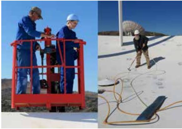
Fig. 3 The surface of the 15-m antenna under repair: vacuum and fiberglass curing in progress. Visiting scientists beware—you will be put to work!
