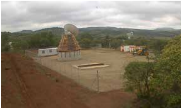
Fig. 4 VGOS site, 15 December 2016; last concrete pour of antenna tower is scheduled for the end of January 2017.
