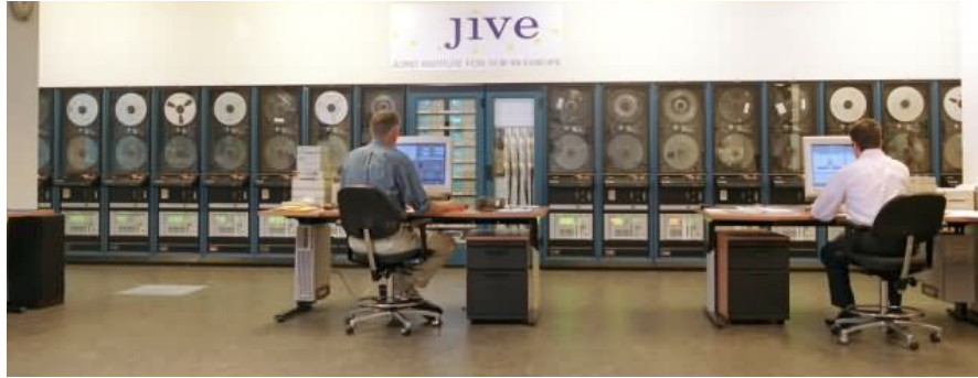
Figure 1. A view of the main control space for the JIVE Mark IV Data Processor.
